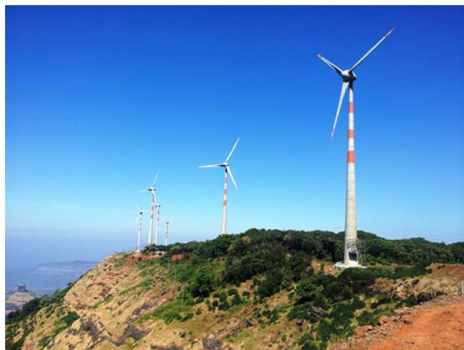
Andhra Lake I Wind Farm offline sales
