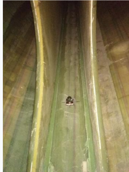
Ventus wireless and battery powered sensor node located inside the blade
